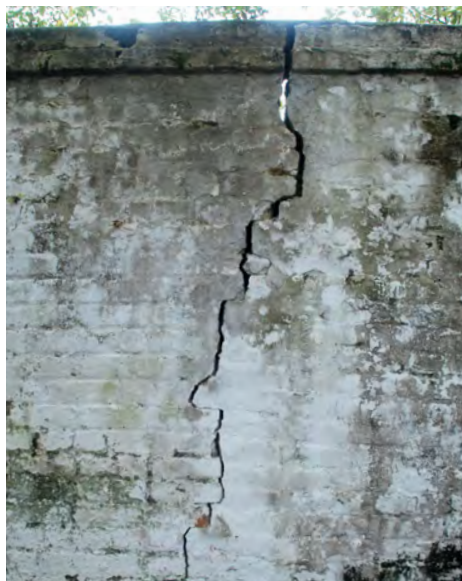
D2: A large crack has formed in this section of the wall.
