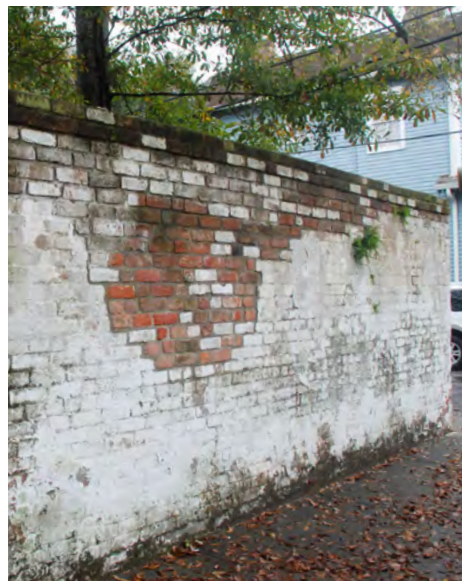
C5: Perspective view showing the recent wall repair along Sixth Street. Some recycled bricks (in white) were used for the repair.
