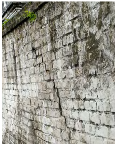
C2: A crack has formed in this section of the wall.
