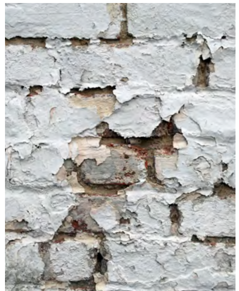
C3: Multiple coatings of paint in various shades of white are visible. The paint is flaking off, exposing weak mortar joints in need of repointing. This condition is prevalent along much of the Sixth Street wall.
