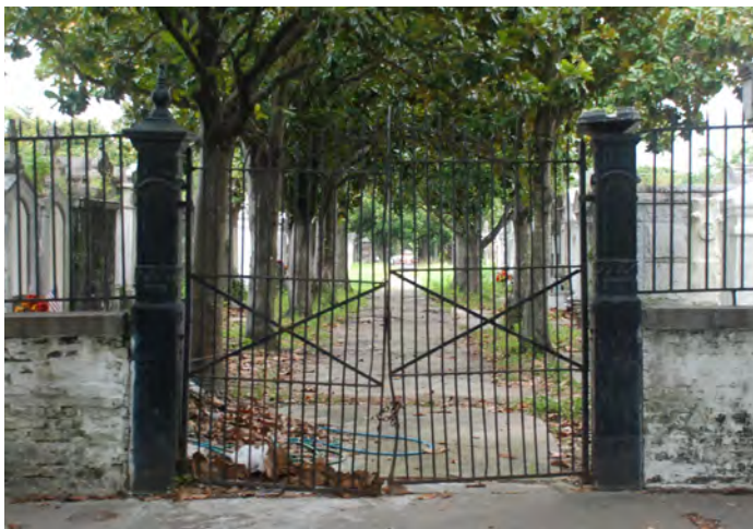
Fig. 24: The Coliseum Street gate is in need of repair.
