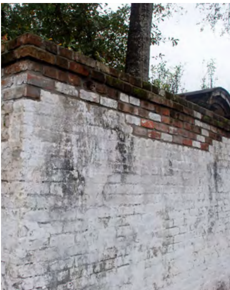
D1: Perspective view showing the recent wall repair along Coliseum Street. Some recycled bricks (in white) were used for the repair.
