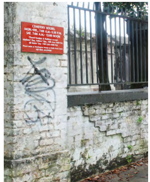
B3: Graffiti, cracks, multiple layers of coatings, mortar issues, and unwanted vegetation are all present in this area near the Prytania Street gate.
