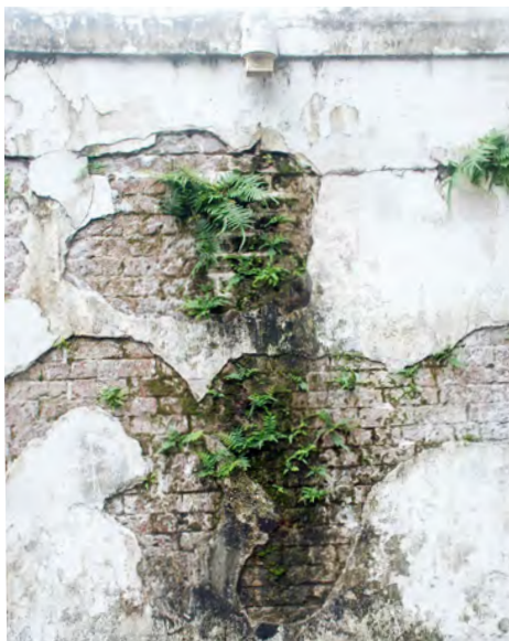
A4: Vegetation growing beneath one of the wall vault roof drains, suggesting that moisture is being trapped.
