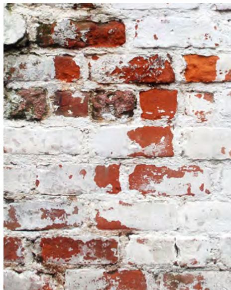
A5: Spalling of older, softer brick (i.e. surface chipping and flaking) due to the use of inappropriately hard cement-based mortar for repointing.
