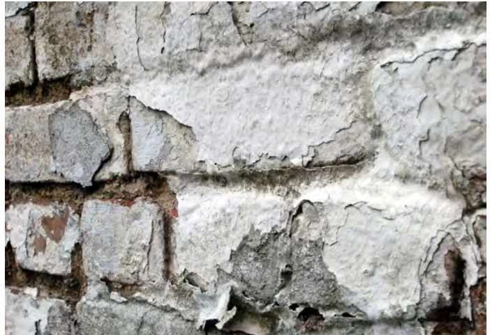
Fig. 19: Detail of the brick wall along Prytania Street showing multiple layers of peeling paint
