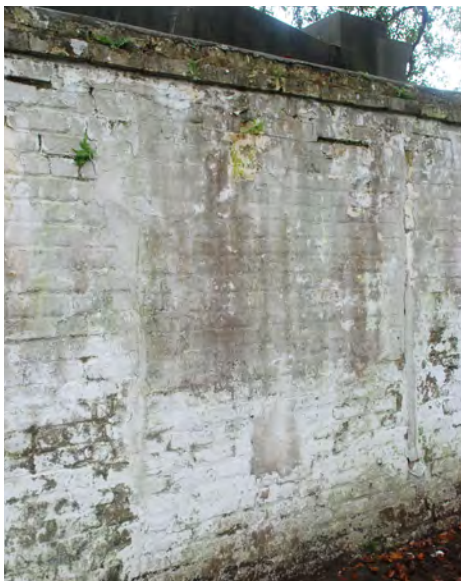
C4: Area of a prior repair. Two vertical cement “seams” are visible.
