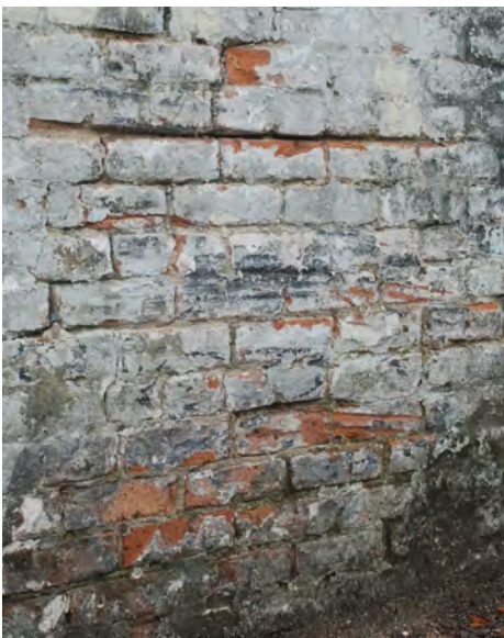
B1: Area where a car appears to have impacted the brick wall.
