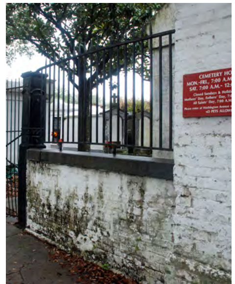
D3: Multiple coatings of paint along with biological growth are present.
