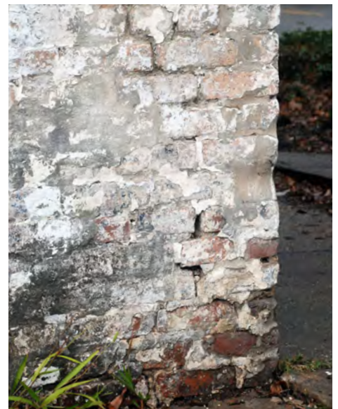
D6: Mortar joints at the corner are in need of repointing.
