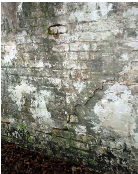
D4: Cracking and bulging, along with the presence of biological growth, suggest the presence of trapped moisture. It is also possible that tree roots could be growing within the brick wall.
