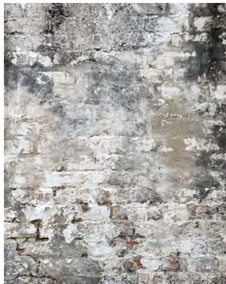
D5: Poor repointing shows several of the bricks smeared with mortar.
