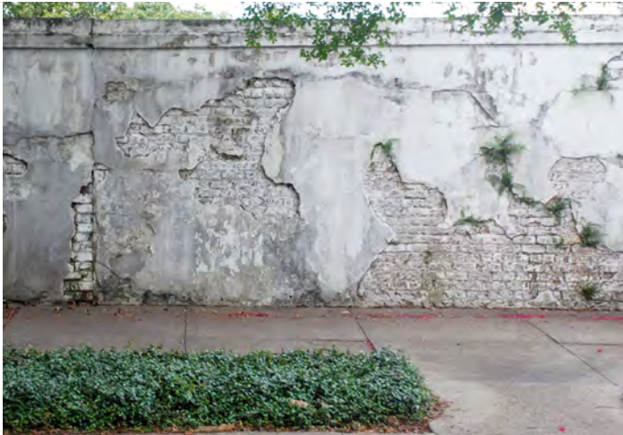
Fig. 20: Detail of the Washington Avenue wall where the cement stucco is gradually being removed
