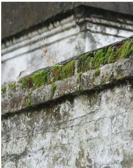
C1: Moss is growing along the top edge of the brick wall.
