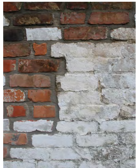
C6: Detail where the recent repair (left) meets the existing brick wall (right).
