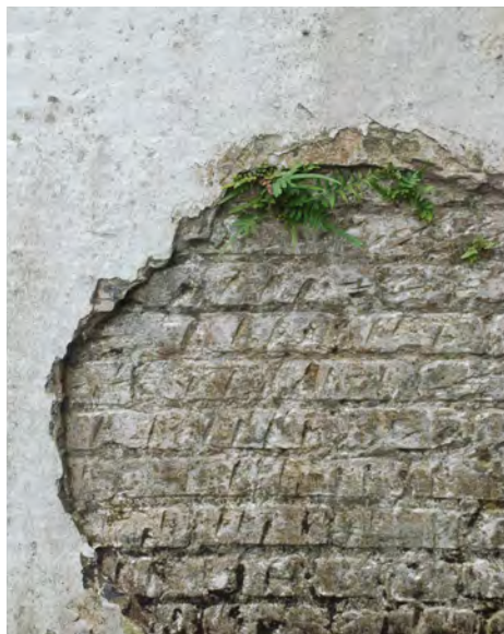
A2: The surface of the brick wall was hatched for better adhesion of the cement-based stucco (which is in now being removed in phases).
