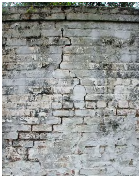
B2: Structural cracks have formed in this section of the wall.
