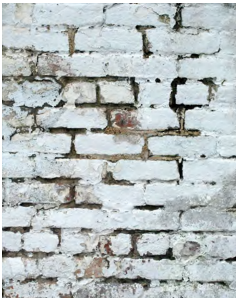
A1: Section of brick in need of repointing. The mortar is disintegrating, providing opportunities for water to infiltrate the wall.
